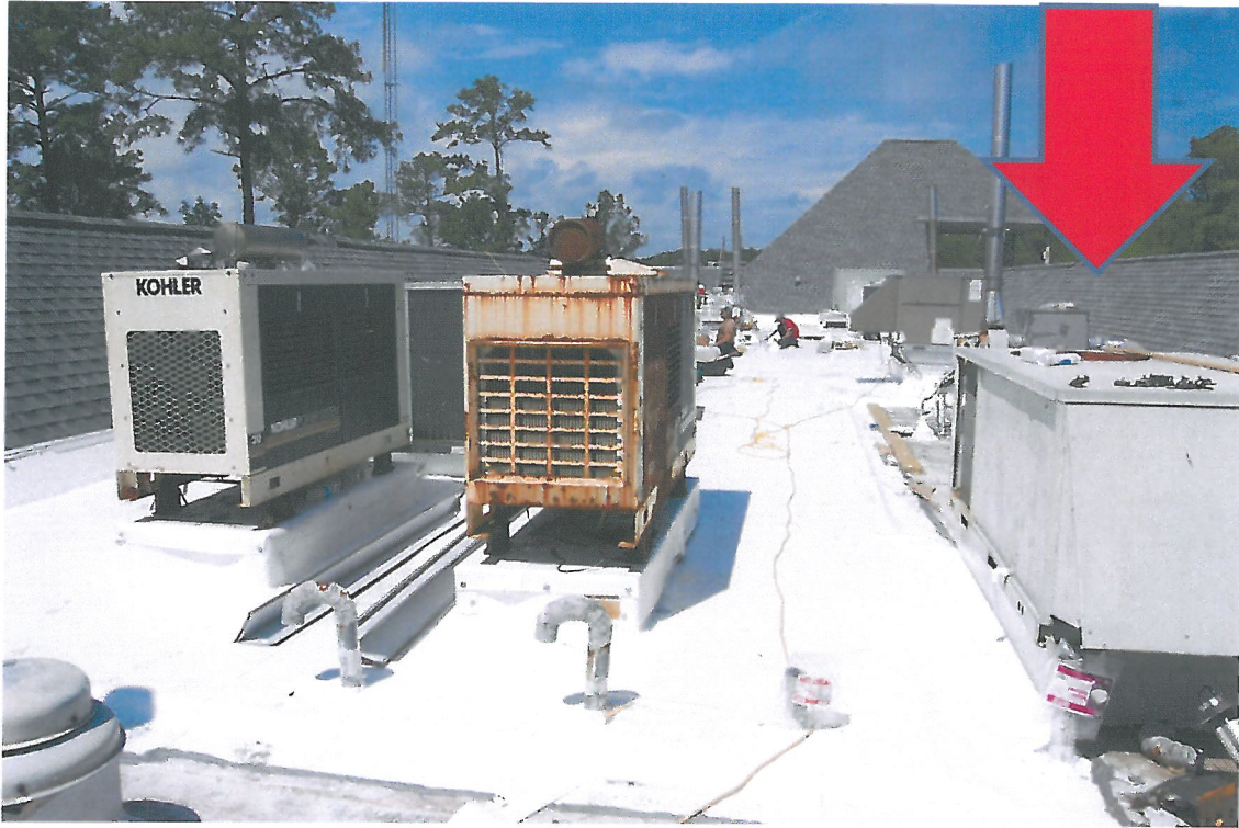
Existing 7.5 ton to be removed and replaced with new 10 ton HVAC unit
