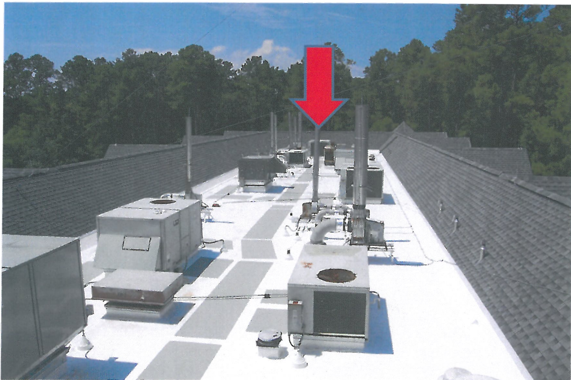
OVER HEAD VIEW OF MECHANICAL WELL ON ROOF. RED ARROW SHOWS HVAC LOCATION
